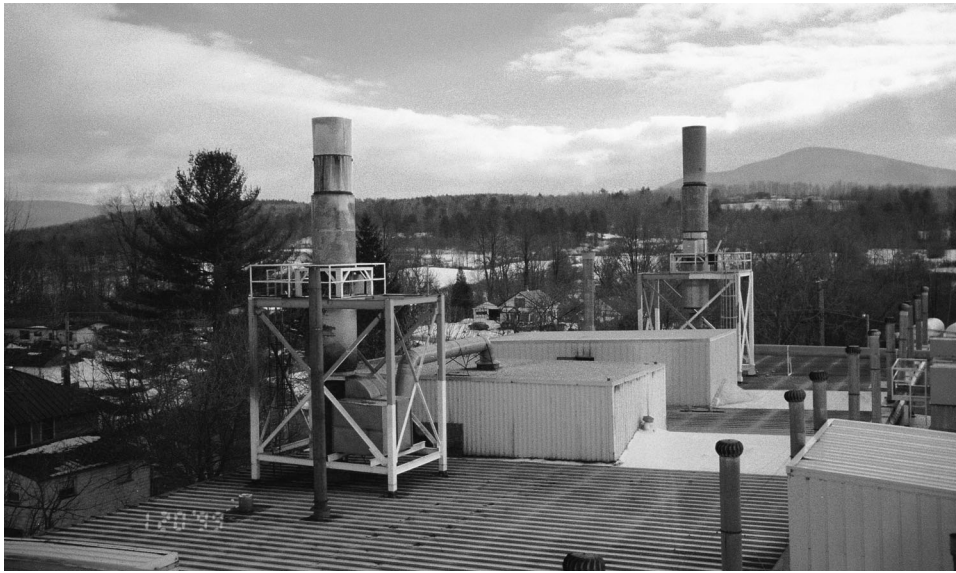
Figure 1. Image from a state inspection of the ChemFab Plastics Factory in Bennington Vermont, January 1999. (Vermont Department of Environmental Conservation)
